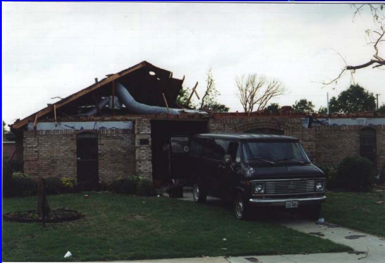
FR12: DOD6: Large sections of roof removed; most walls remain standing
